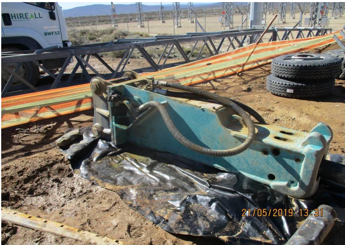
Photo: Excavator packer is placed on the bare ground without effort/measure in place to prevent soil contamination
