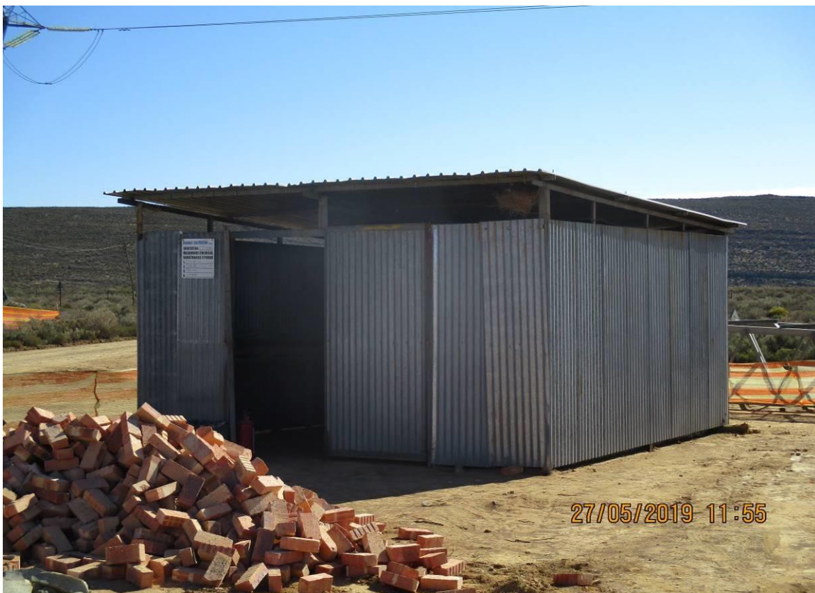
Photo: Hazardous store that does not meet the minimum requirements.
